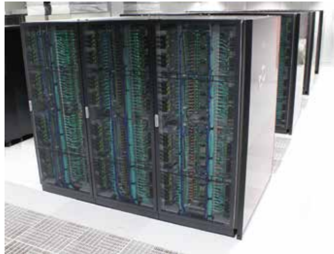
▲HPC System (TOKI-SORA)
